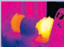
Overheating bearing cap
